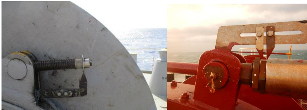
Fig 11: Mooring Winch Brake Correct Setting/Alignment.
