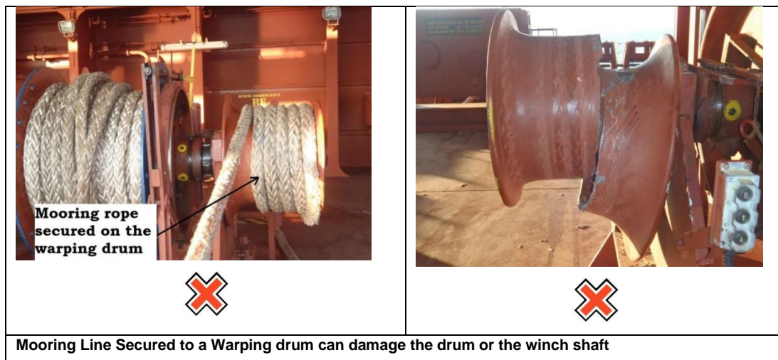
Fig 12: Mooring Winch Line secured to warping drum. (Source Anglo Eastern)
