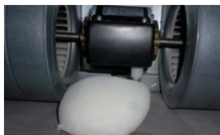
Duct Air Treatment in Ducted Unit
